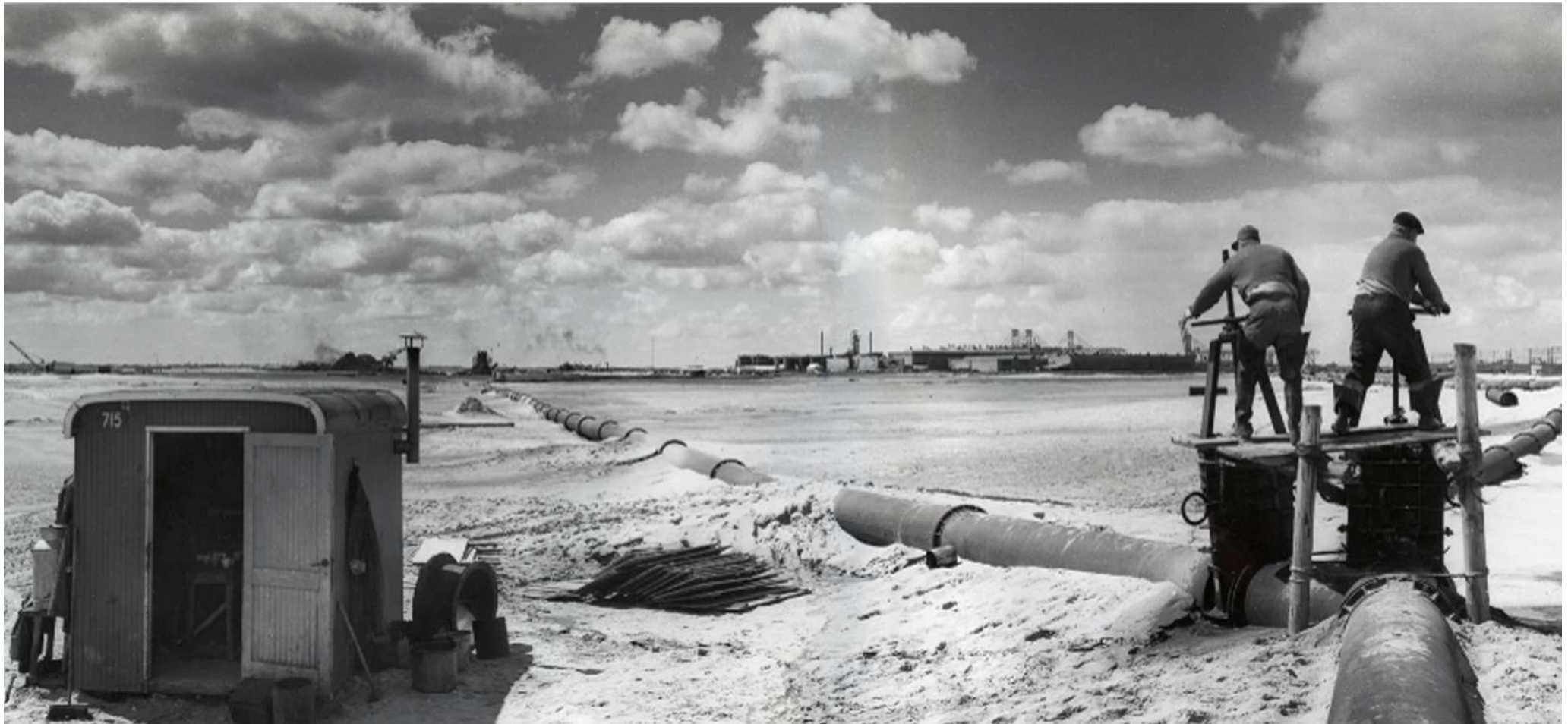
Pumping 4+ meters of sand on the southern IJ-river shores for the new ports of Amsterdam (1963)
